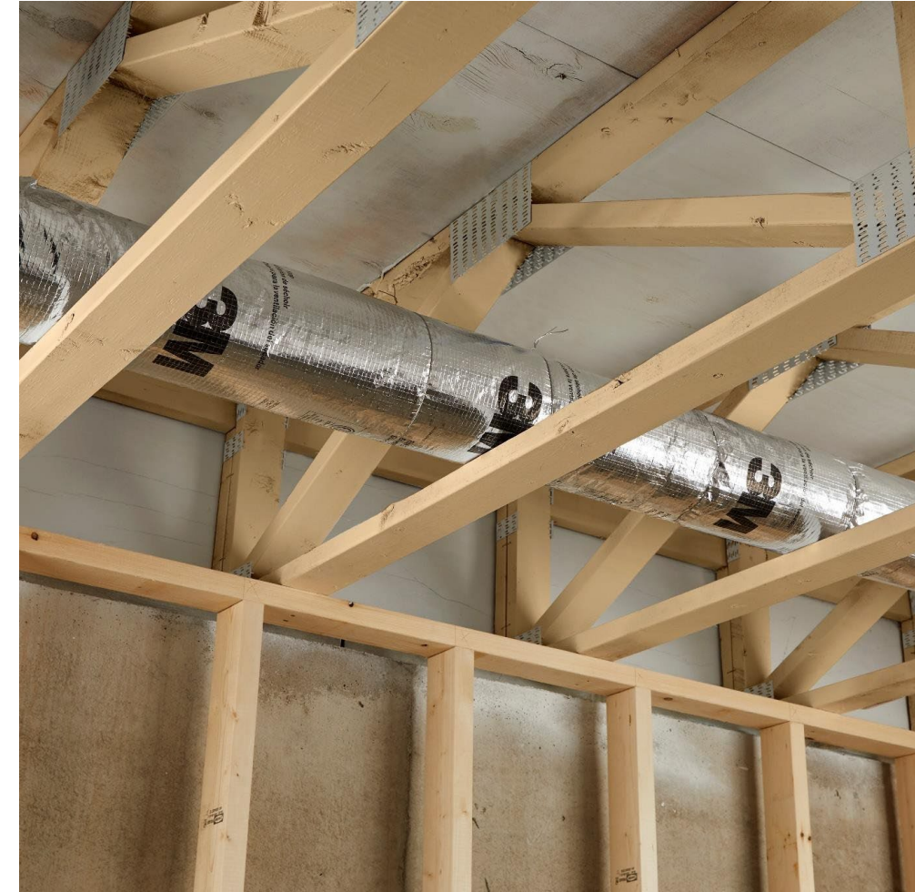
Dryer ventilation wraps
