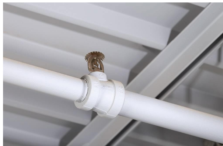
Sprinklers Fire Departments
